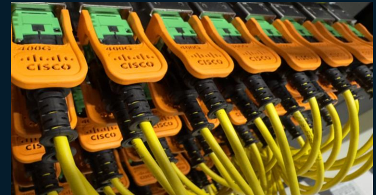
Cisco's QDD-400G-DR4-S 400G optic providing network connectivity on the Network side for AI cluster's non-blocking Compute fabric
