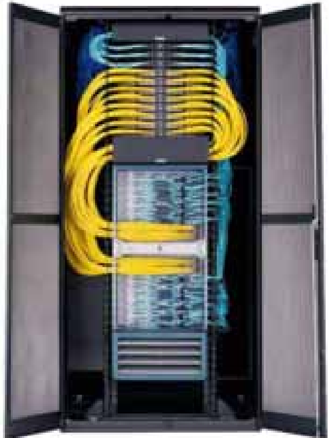
Net-Access™ N-Type Cabinet with Cisco^ Nexus 7018 Expansion Module Installed
