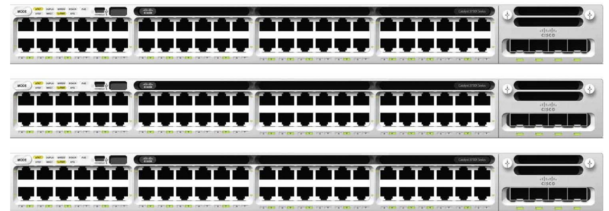
Next-Generation Switches (Catalyst 3850s)
