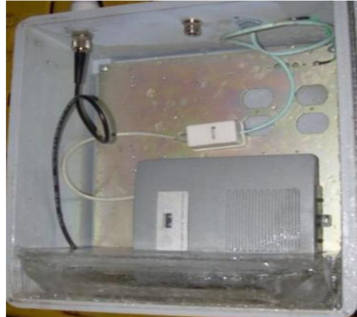
Outdoor NEMA box not weatherised (just keeping the packets on ice)
