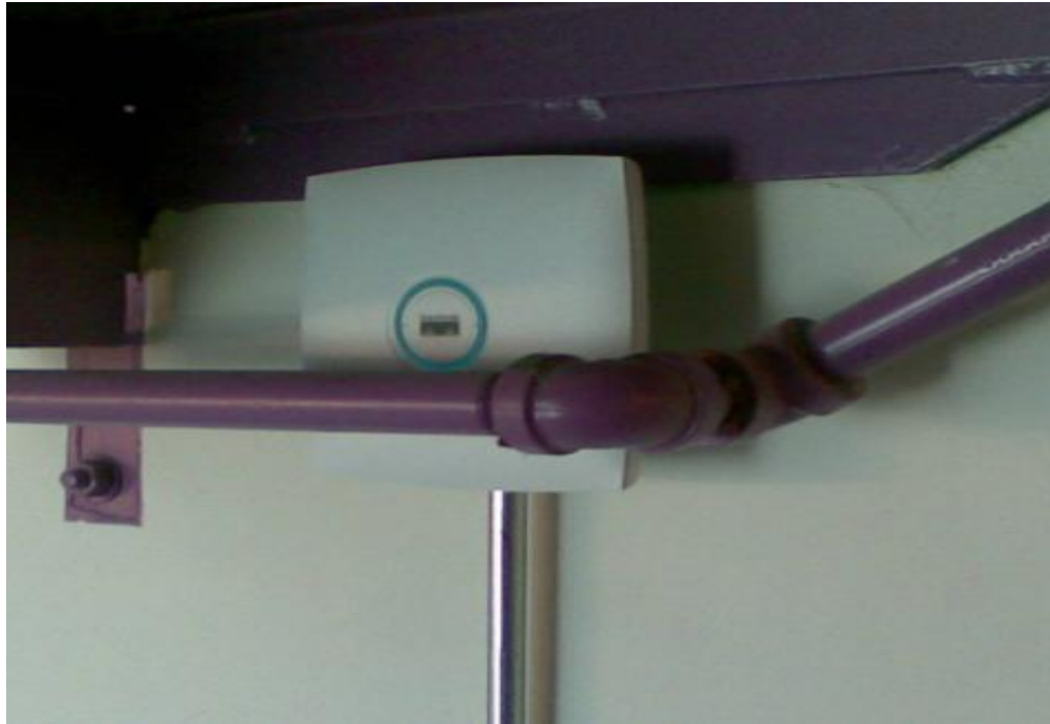
Ceiling mount AP mounted on the wall up against metal pipe (poor coverage)
