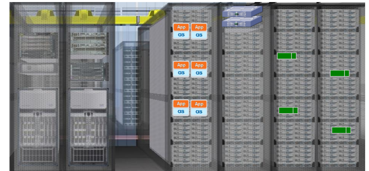
Data Centre Row 2
