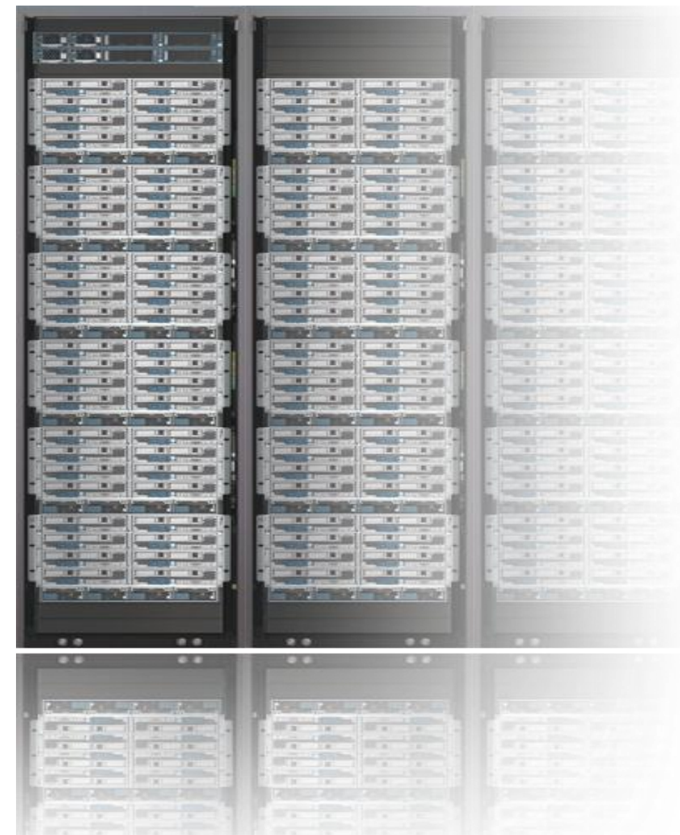
Virtualised Multi-tenant Data Centre
